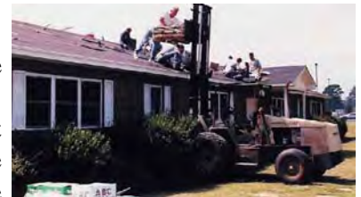
A much needed roof is installed on the Little People's dorm at the Children's Home by workers from White Savannah FWB Church, Oak Grove FWB Church, and North Conway Church of God
